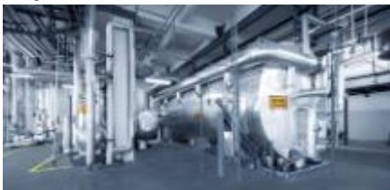
Fig. 1: Continuous Polycondensation: Total Control over the entire process chain.
