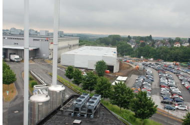
Caption: The view from above of the construction site on Leverkusenstrasse in Remscheid Lennep – the new pump manufacturing production building of Oerlikon Barmag.
