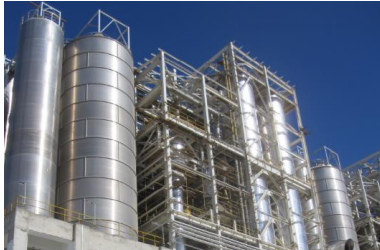
Fig. 1 The turnkey plant was handed over to EIPET at the beginning of 2014.
